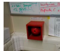
Electrical stop of this room
