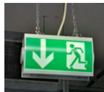
Sign for emergency exit
