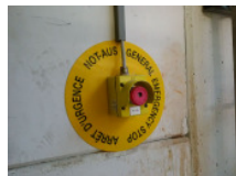
Button for power emergency stop
