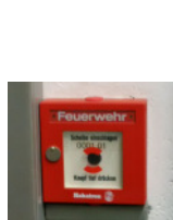
Fire alarm button
